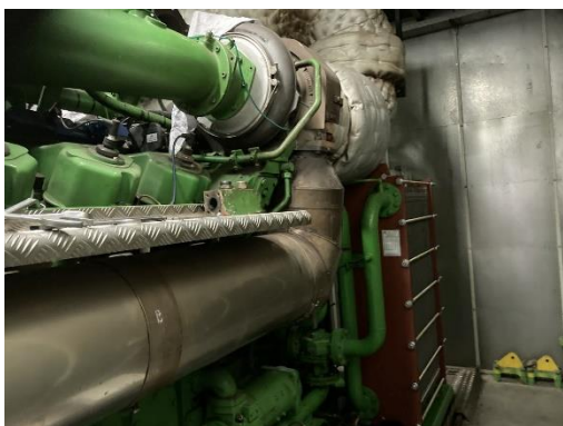
Part of a CHP unit
