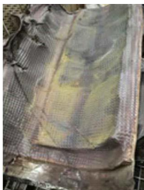
Yellow dust deposits beneath section of insulation
